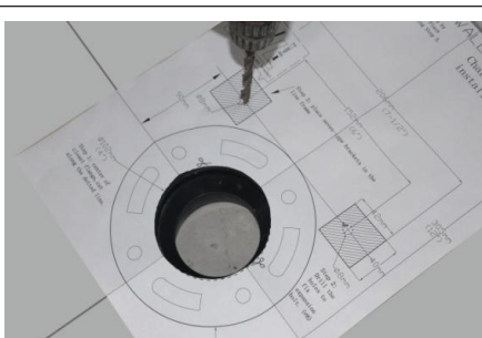
5. According to the instructed location in the instruction, drill two holes (diameter of which is 8 mm) for the floor screws.
